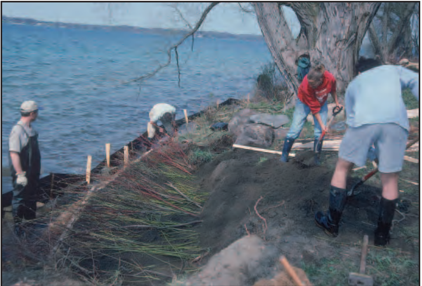
Volunteers construct a vegetated geogrid for a demonstration project at MSU's Kellogg Biological Station on Gull Lake
