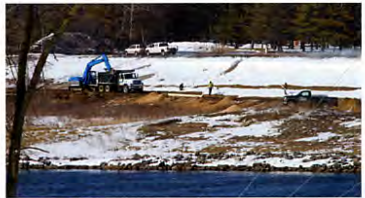
Crews continue to make repairs to the Sanford Lake dam in Sanford. The water levels have been lowered so crews can make much needed repairs to the berm portion of the dam.
